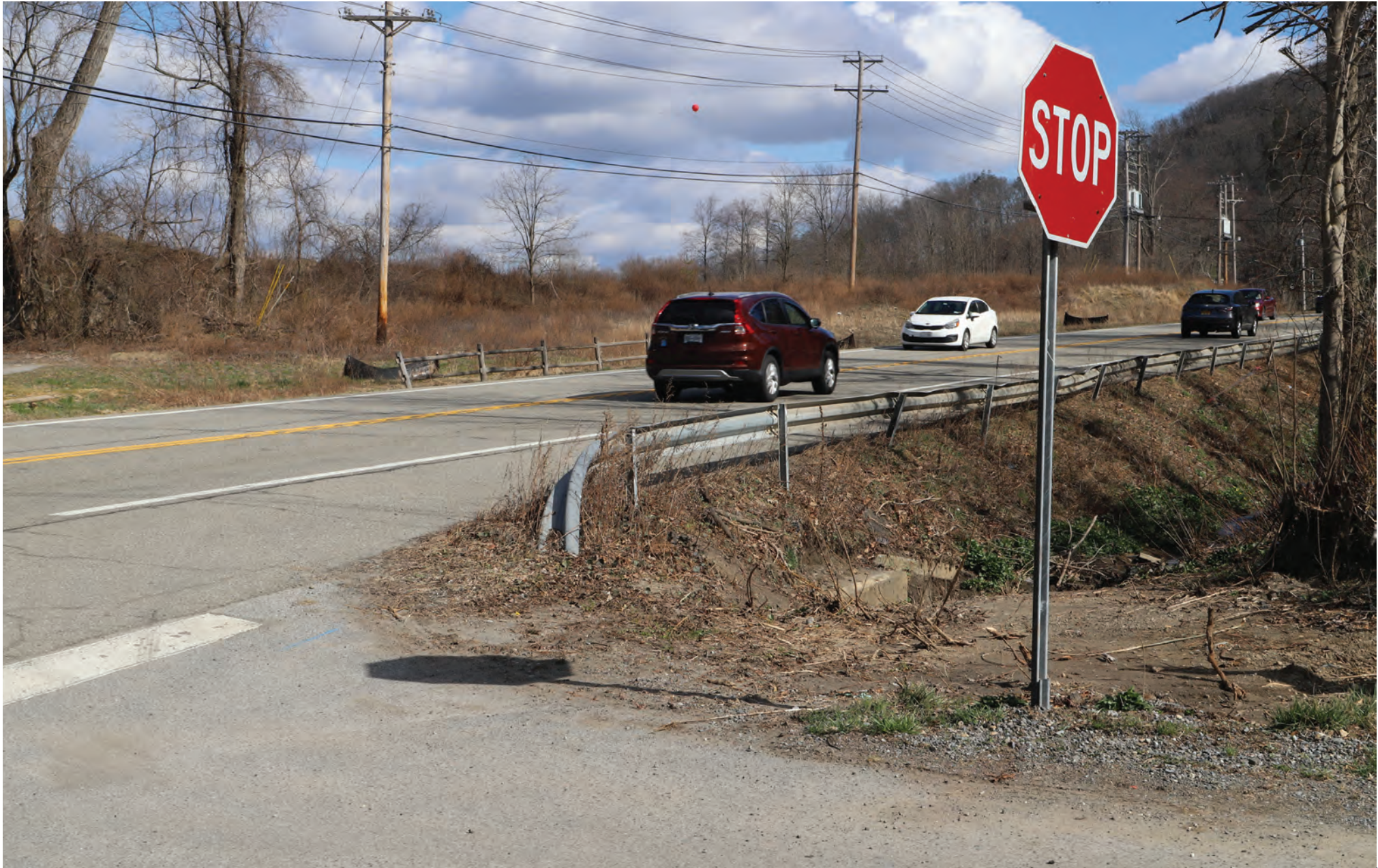
Photo 16 - NY Rte. 9 at Carol Lane EXISTING CONDITION
