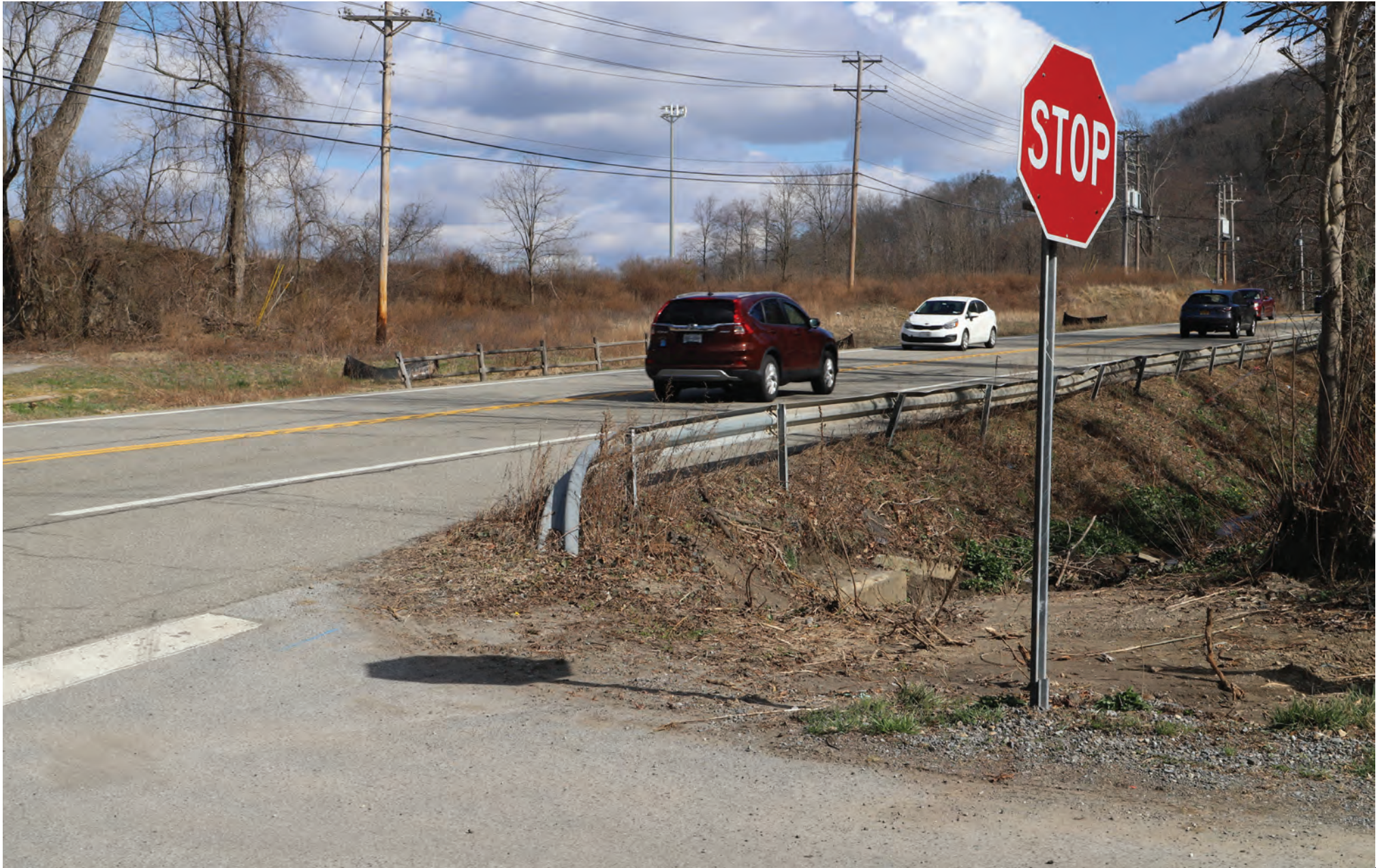
Photo 16 - NY Rte. 9 at Carol Lane SIMULATED CONDITION - Galvanized Steel Option
